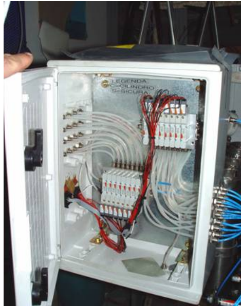
Figure 3: The watertight box containing the electro-pneumatic valves feeding the pneumatic actuators.
